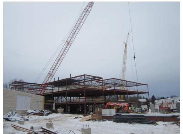
The steel structure of the 6 th , 7 th , & 8 th grade wing is moving west.
