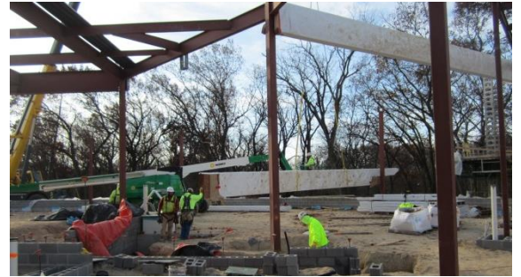
Crews have begun the installation of the timber beams in the cafeteria.
