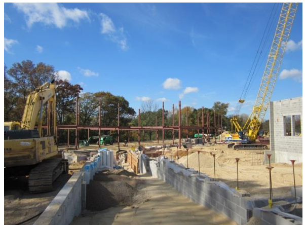
Looking down the corridor from the cafeteria the installation of the structural steel of the 6 th , 7 th and 8 th grade wing has begun.
