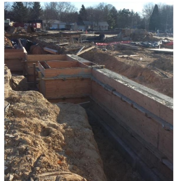
Footings and foundation walls. This will become the north wall of the new gym.
