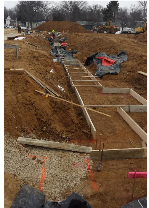
The foundation wall above will form the east wall of the new gym.
